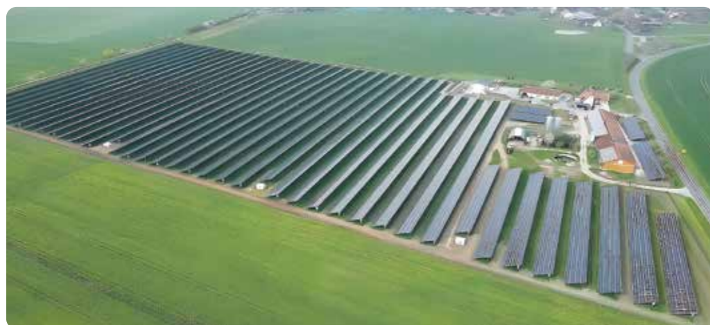
11.2MW Bavaria, Germany
